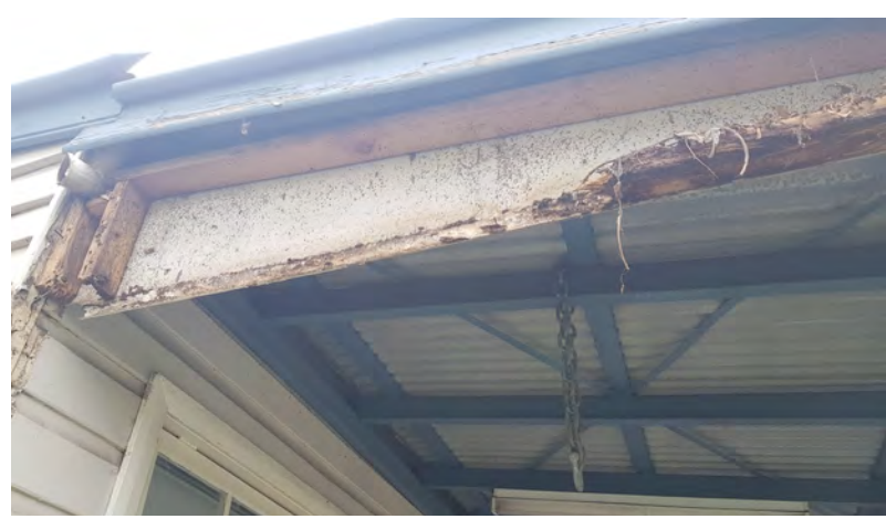
IMAGE 6: PHOTO OF DILAPIDATED CONDITION OF EXISTING REAR AWNING
